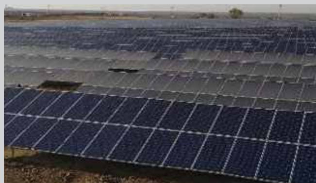
Axis Bank's 2 MW ground-mounted solar power project at Solapur, Maharashtra
