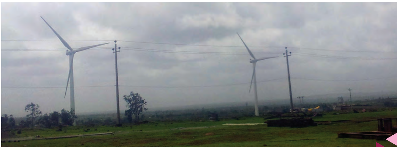
Windmill installed at Doddanavar Global Energy
